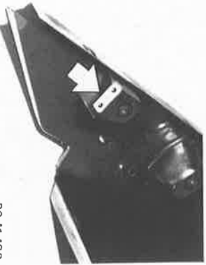
Drill holes for plug spot welding in holder for engine hood lock.
